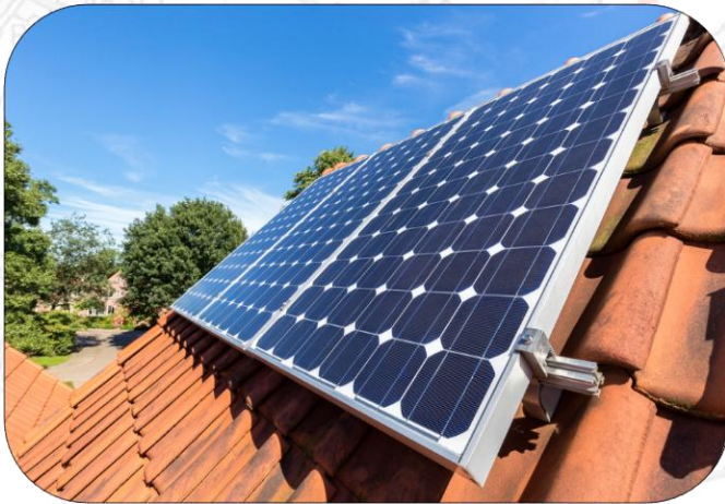
Rooftop Solar PV
