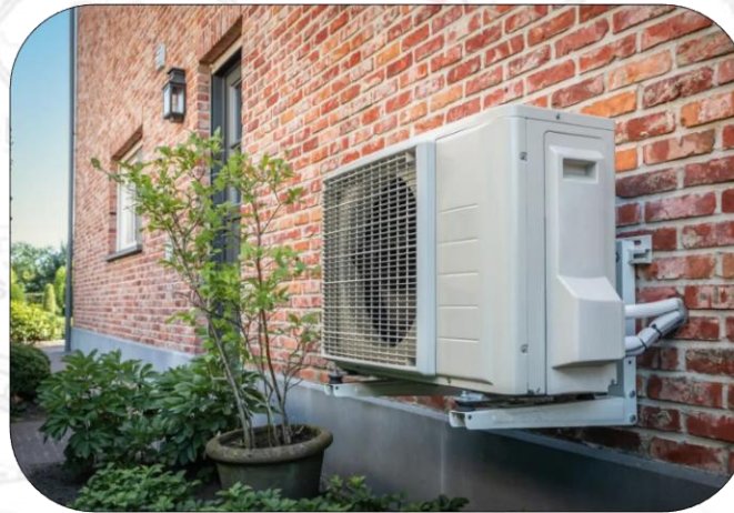
Domestic Air- Source Heat Pumps
