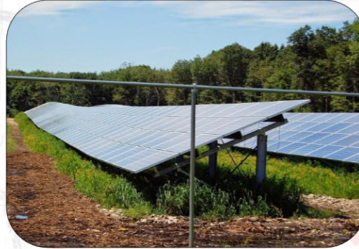
Solar PV (ground)
