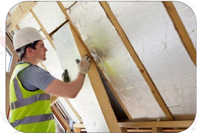
Domestic Energy Efficiency Measures
